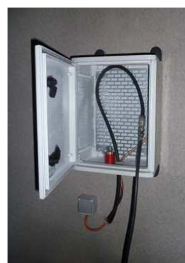
Coffret tunnel TGV
