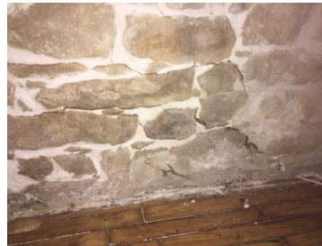
Fissuration de traction
